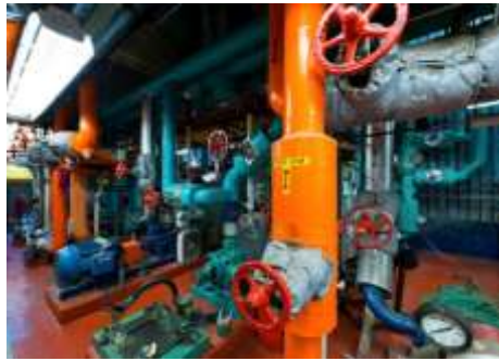
Steam to Hot Water Conversion of Campus District Energy System
