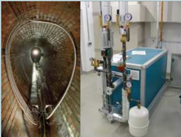
Waste-Water Heatpump (2 x 22 kW)
