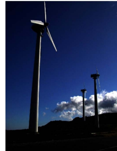
Ikaria: 4.5 MW wind, 2.73 MW hydro, 1.04 MW PV, 15.85 MW diesel
