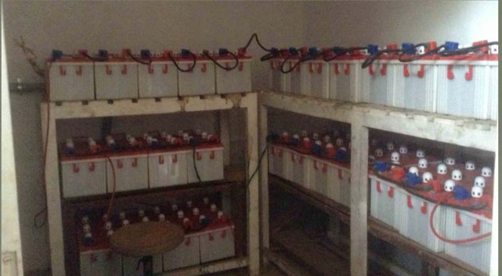
A battery system backing up City Hall in Auroville (photo C. Eggleston)
